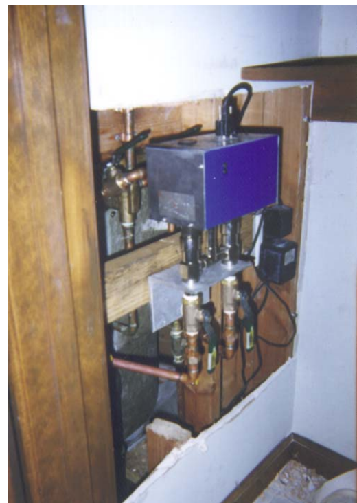
Figure 17.36. Installed Water Temperature Adjustment Control System.
