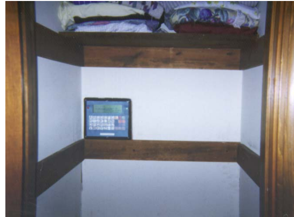
Figure 17.35. Installed Front Panel of the Water Temperature Control System, Mounted in a Closet that Backs up to the Shower Plumbing.
