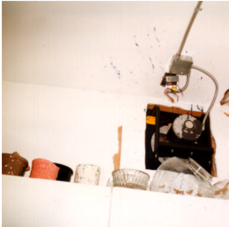
Figure 7.5. Installed Fan Shown From Interior.
